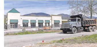
A truck drives past construction at the base of the property of the Black Mountain Home for Children, Youth and Families on April 18. The building will be a thrift store and cafe to benefit the home. ANGELI WRIGHT/AWRIGHT@CITIZEN-TIMES.COM
